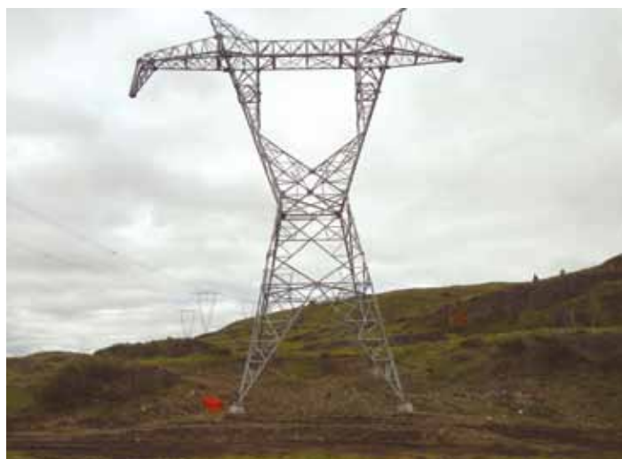
Credit: BC Hydro
